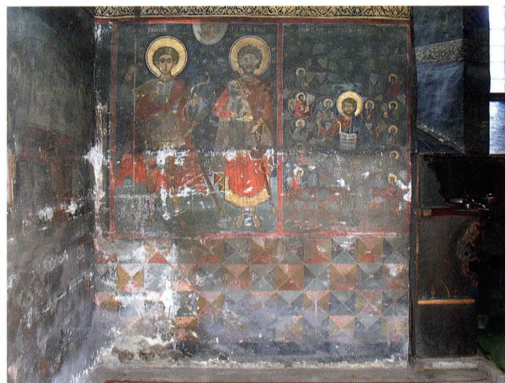
Fig. 16. Nave. Murals damages due to erosion
