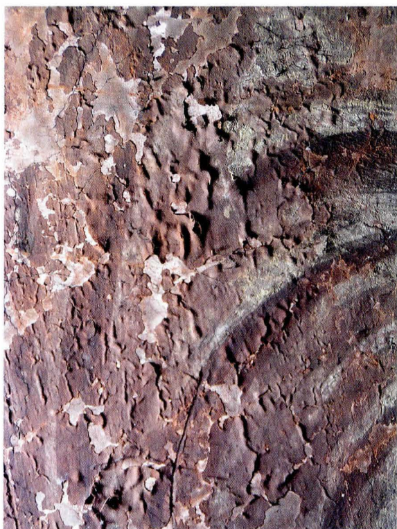
Fig. 26. Loss of adherence of the paint layer
