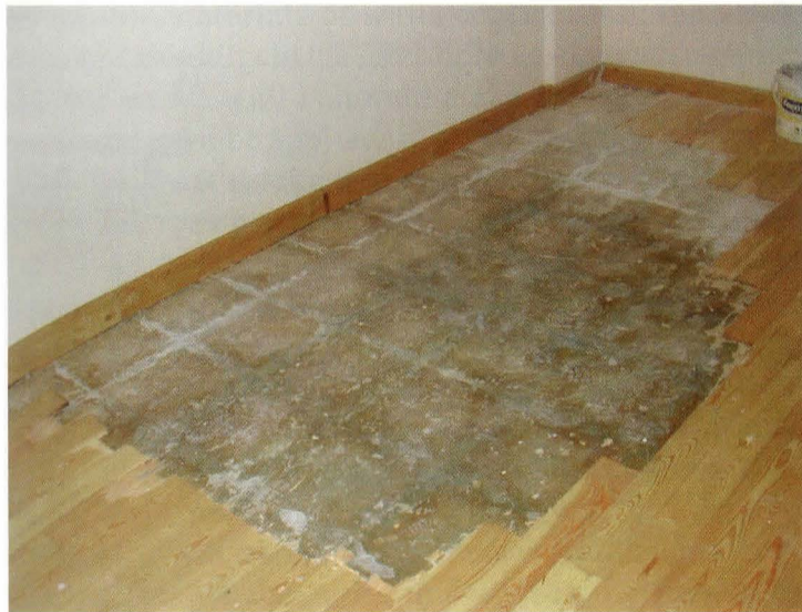
Fig. 2. Damage floor due to humidity
