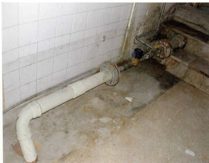
Fig. 14. Water supply pipes with leaks
