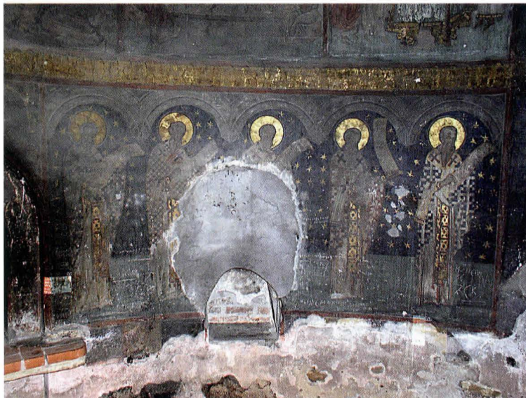
Fig. 13. Chancel. Inside. Degradation and loss of the painting due to capillarity moisture
