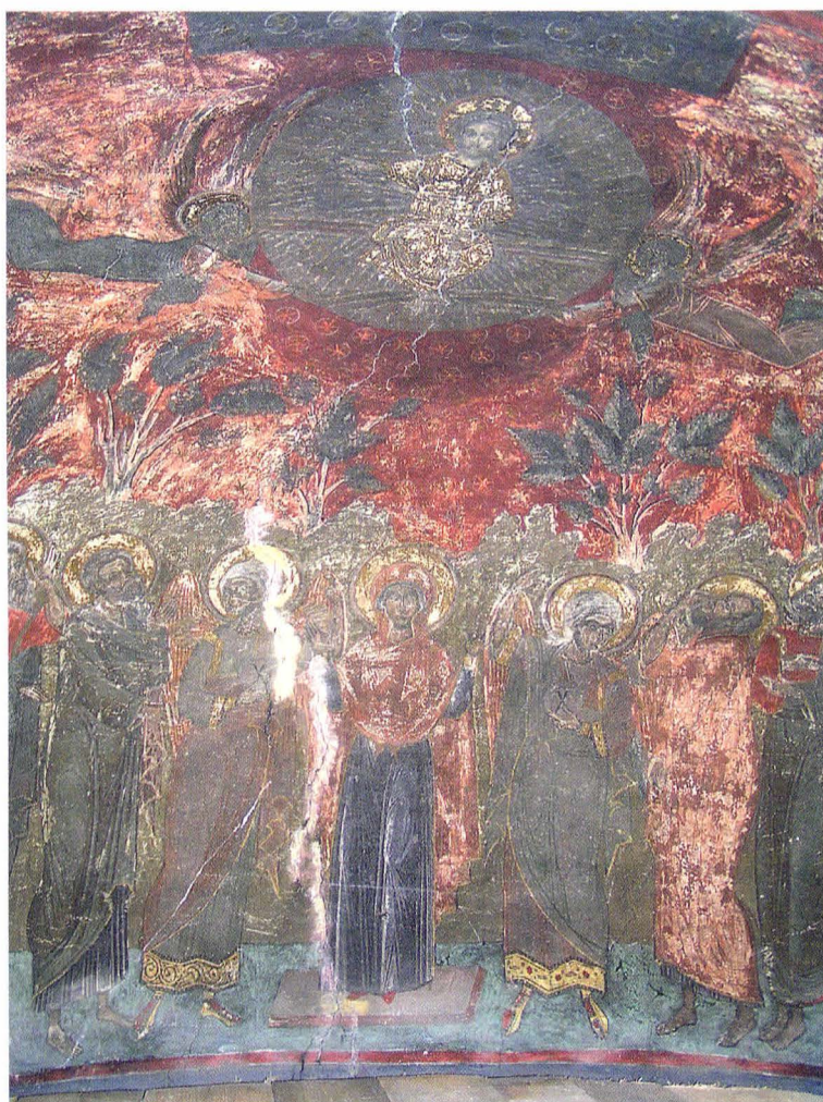
Fig. 15. Chancel, semicupola. Cracks and detachments
