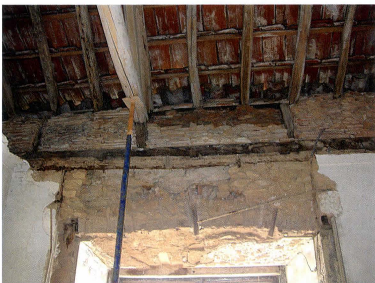
Fig. 11. Damage on structure due to infiltration
