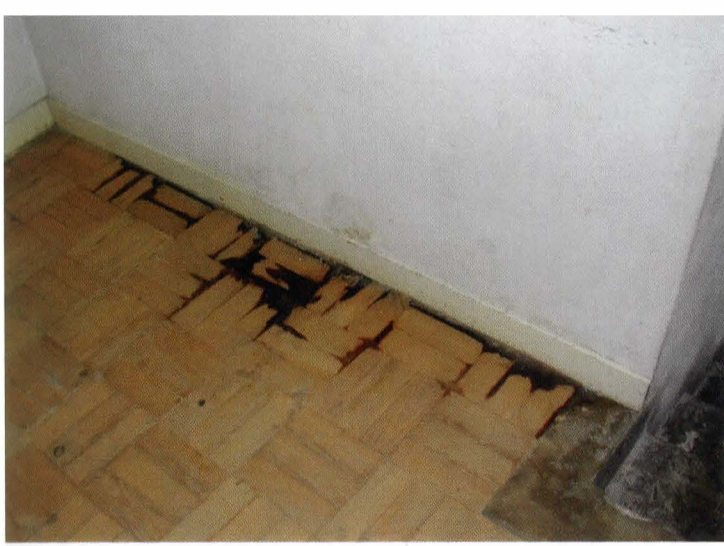
Fig. 1. Humidity in floor
