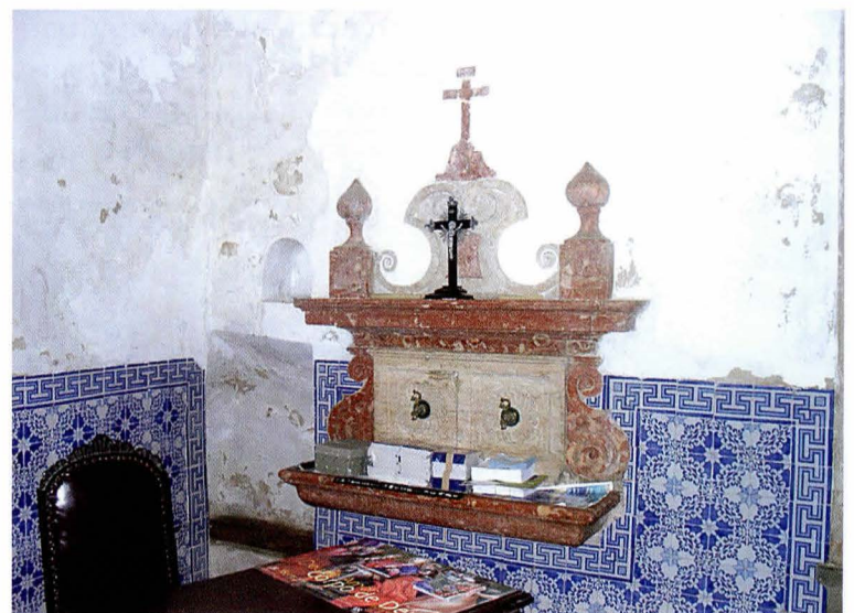
Fig. 15. Efect of condensation water
