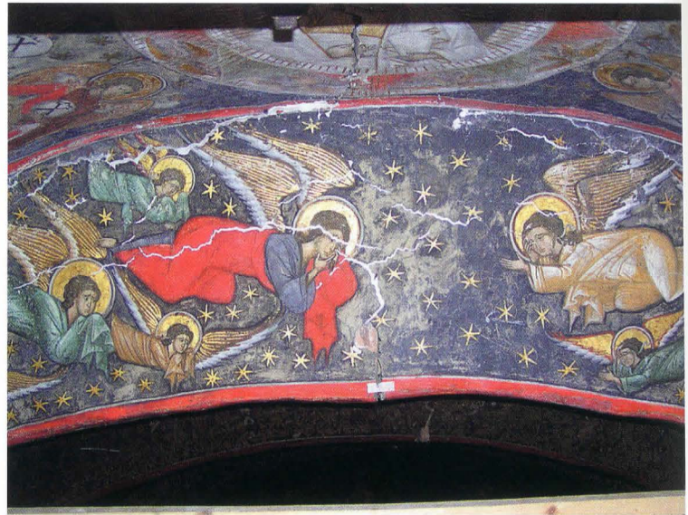
Fig. 13. Triumph arch : cracks and detachments coming from the structure
