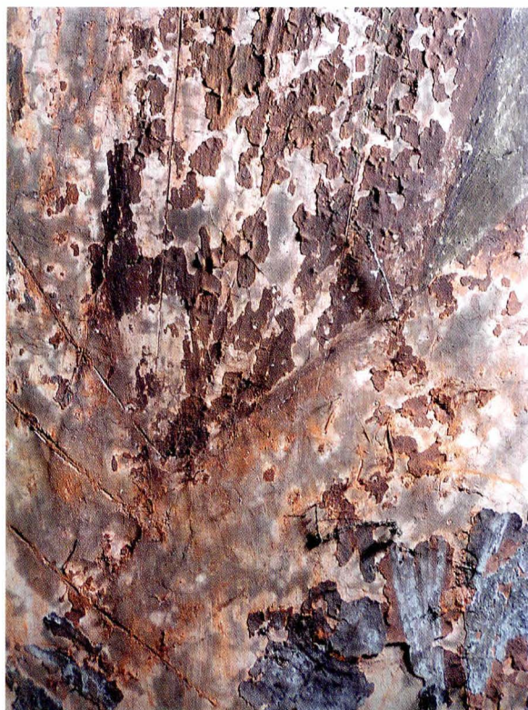
Fig. 27. Loss of adherence of the paint layer
