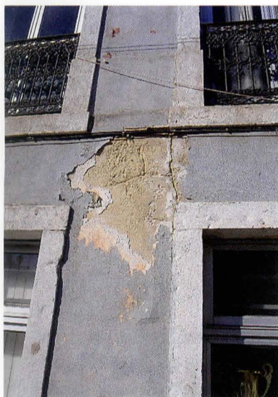
Fig. 9. Loss of paint due to incompatibility of materials
