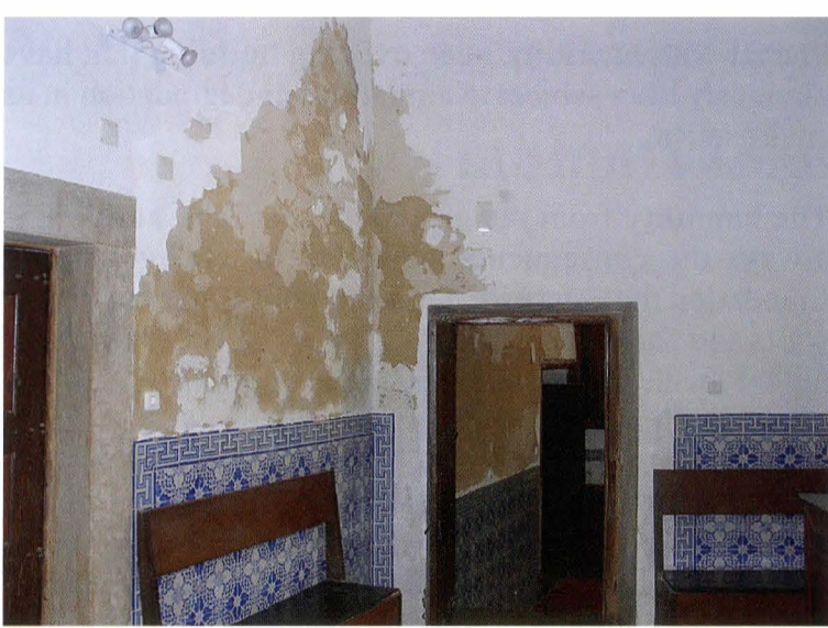
Fig. 5. Damages due to ground humidity
