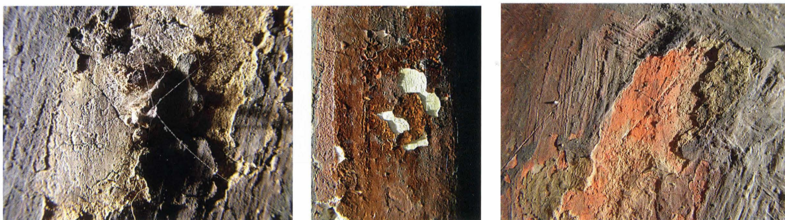
Fig.3. Loss of adhesion of the paint layer in its thickness or on the intonaco support
